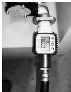
Fig. 6.2.1: Flow meter for 1251 / 2001 tank
