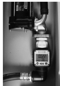
Fig. 6.2.2: Flow meter for 4301 / 4601 / 6001 tank
